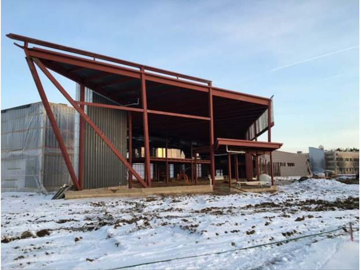
View from near campus flagpoles towards front entrance of the Hanson Technology Center
