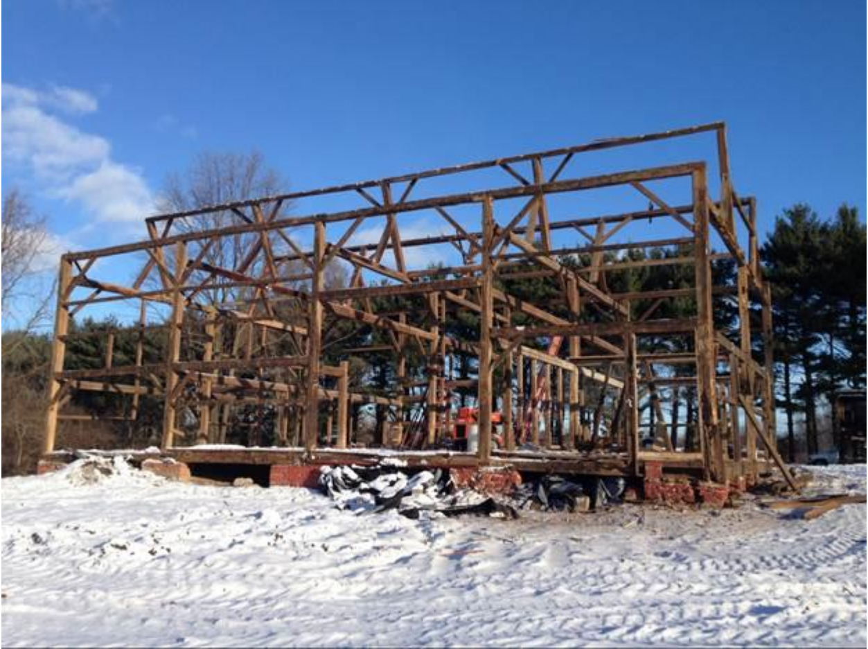
Barn Deconstruction: end of day 2, view from rear of barn looking north
